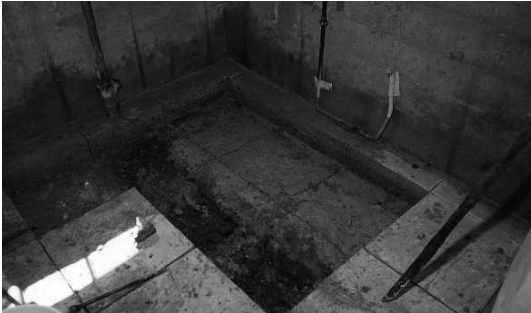
Figure 7. Photograph of void after removal of a portion of the concrete floor.
